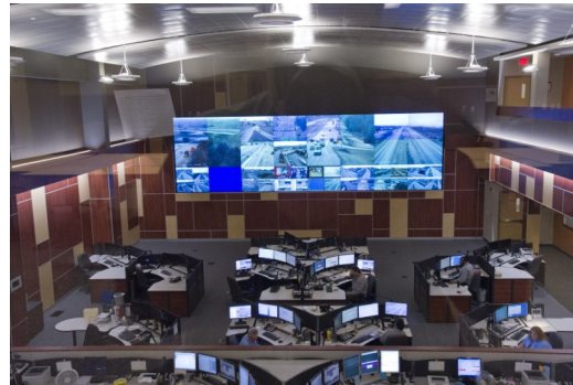
SE Michigan Transportation Operations Center
